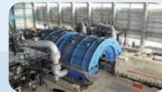
汽轮发电机组 Turbine-generator Unit
